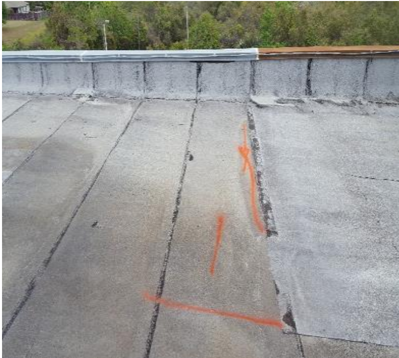
Blister in the roof membrane
