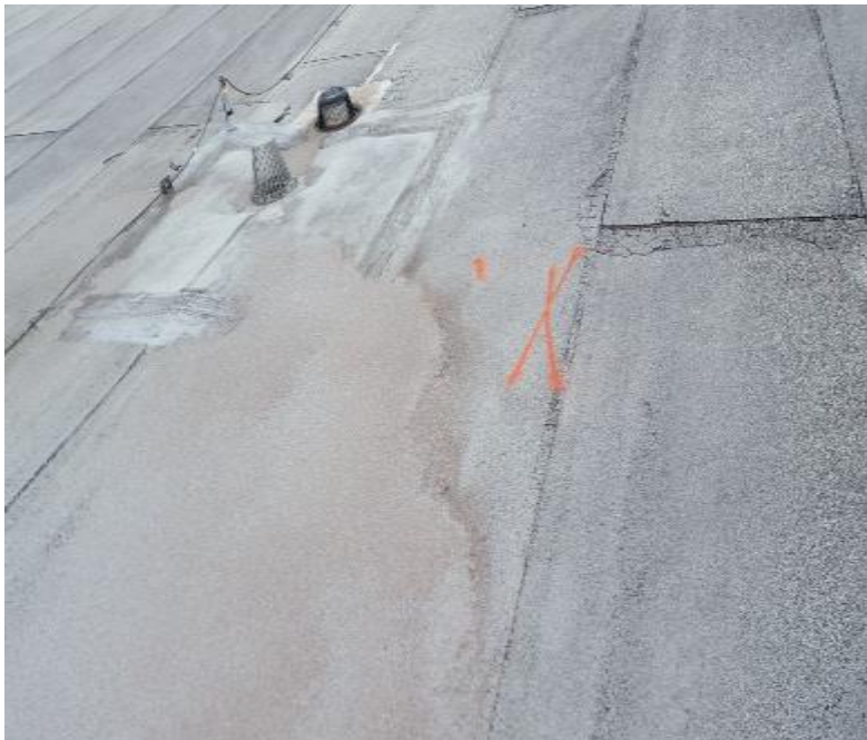
Blister in the roof membrane
