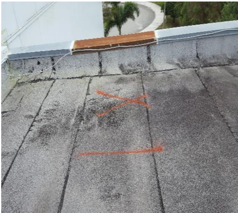
Blister in the roof membrane
